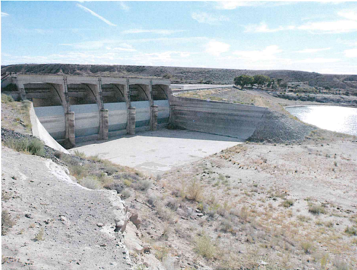
Figure 3. The upstream side of the Rye Patch Dam and Rye Patch Reservoir on the Lower Humboldt River in August 2015.
