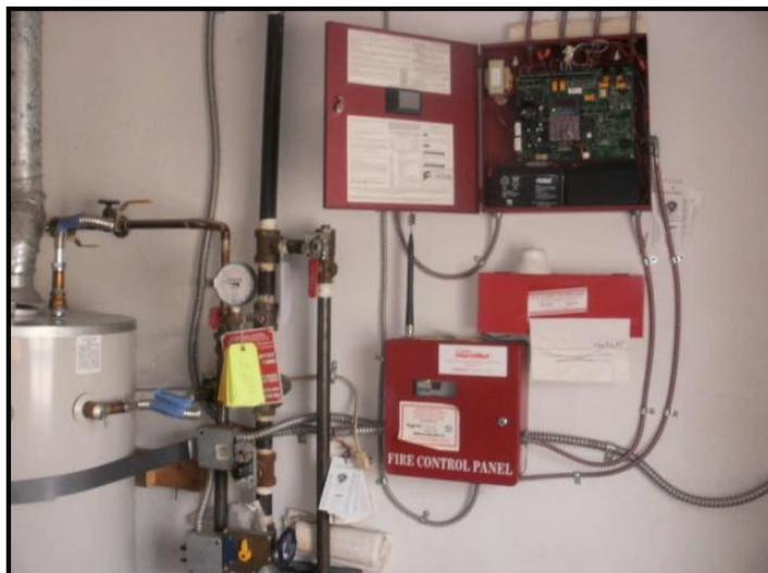
Fire Suppression System
