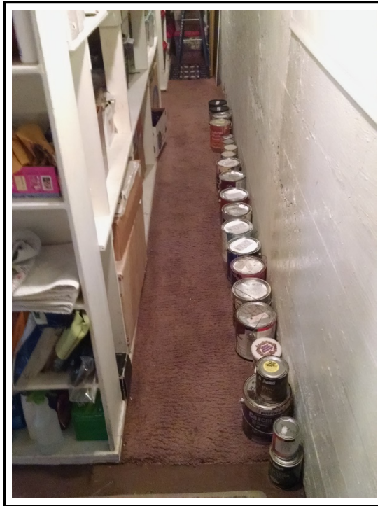
Photograph 5: Paint cans stored in the basement.
