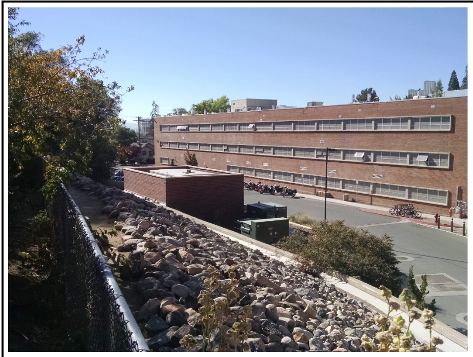
Photograph 7: The diesel-powered electrical generator and electrical transformers located approximately 40 feet southwest of the Subject Property. The UNR Fleishman Agriculture Building is located beyond.
