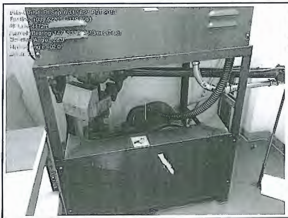
Photograph 16: View of elevator room with operating equipment located in the basement of the building
